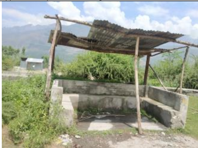
Old damaged Bus Shelter/ Bay coming within the approach of the Srinagar Side.
