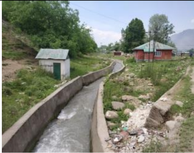
Small Nangdara Irrigation Canal traversing through the approach (LHS) from Srinagar Side. Box Type Culvert is proposed for this Canal.
